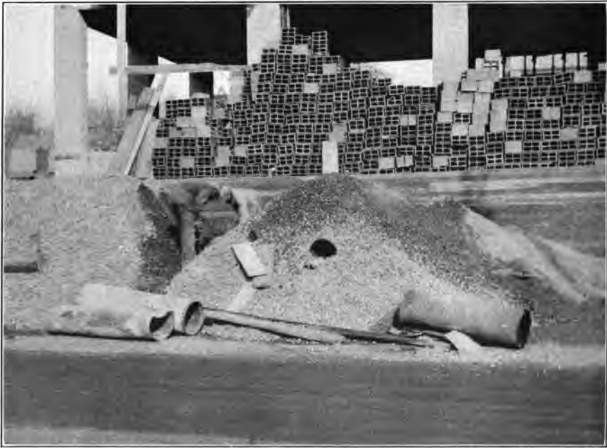
FIG. 5.—HEATING STONE WITH SHEET IRON CYLINDERS. Workmen are digging trench for placing additional cylinders.
